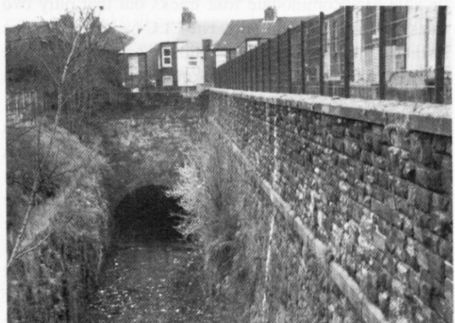
Looking southwest at the northeast portal of Walton-on-the-Hill Tunnel No. 2 which is located in a cutting at Listor Street. The land on the left side of the cutting had been earmarked for a widening of the cutting which would have allowed two extra lines to have been laid. Photo by Paul Wright
